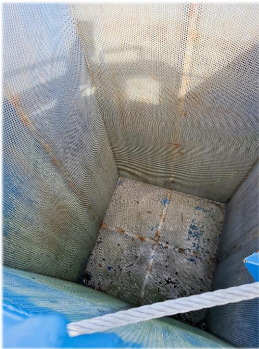
Figure 2- Mesh system inside tank
