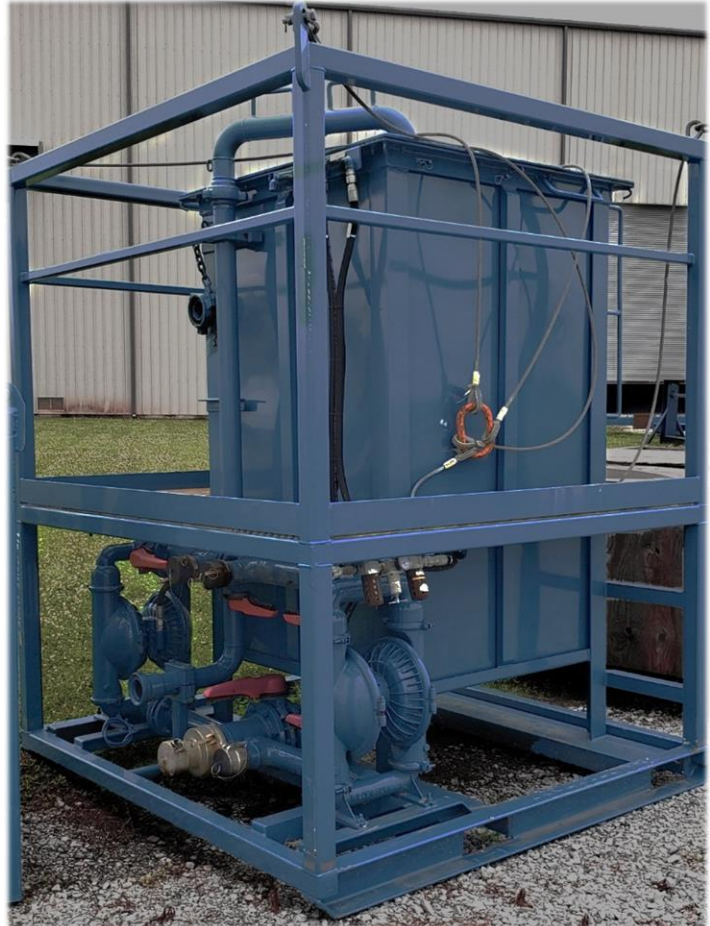
Figure 3- Mixing tank unit with wildem pumps
